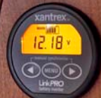
Battery voltage - at high rates of draw the voltage will drop
