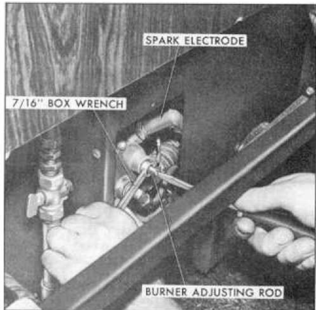
Furnace Primary Air Adjustment
