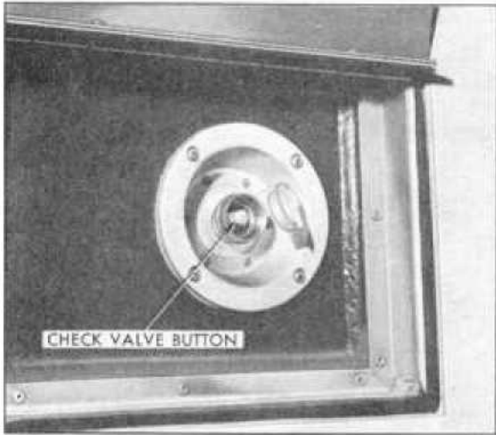
External Water Connection
